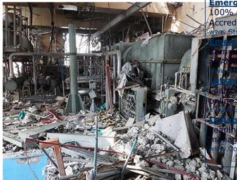
Destruction on the fourth floor of the Fukushima Daiichi Unit 4 reactor building, June 9, 2011 (Photo courtesy TEPCO)
